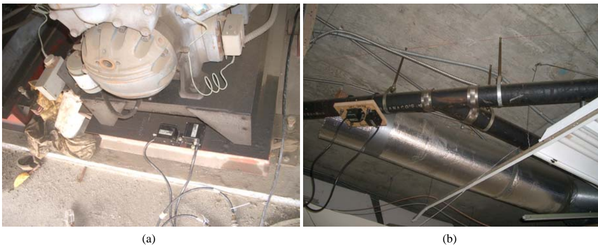
Figure 5. Other nonstructural elements monitored in building: (a) roof compressor and (b) drainage piping system
